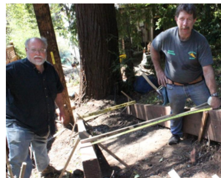
Steve Glaeser (left) and Don Kreiss laying the base lumber for the stairs
